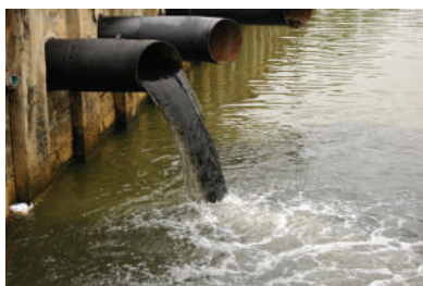
Fig. 12.9: Water contaminated with sewage waste
